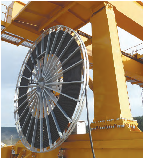
Mono spiral motorised cable drum feeding power to large gantry crane.
